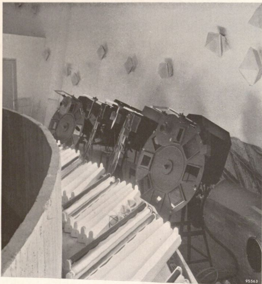
Fig. 5. Glimpse behind the balustrade. Some of the variously coloured fluorescent lamps can be seen and, behind them, an array of projection lanterns with filters for the "ambiances". Above, on the wall, a number of high-note loudspeakers with filters. Bottom right a low-note loudspeaker.
