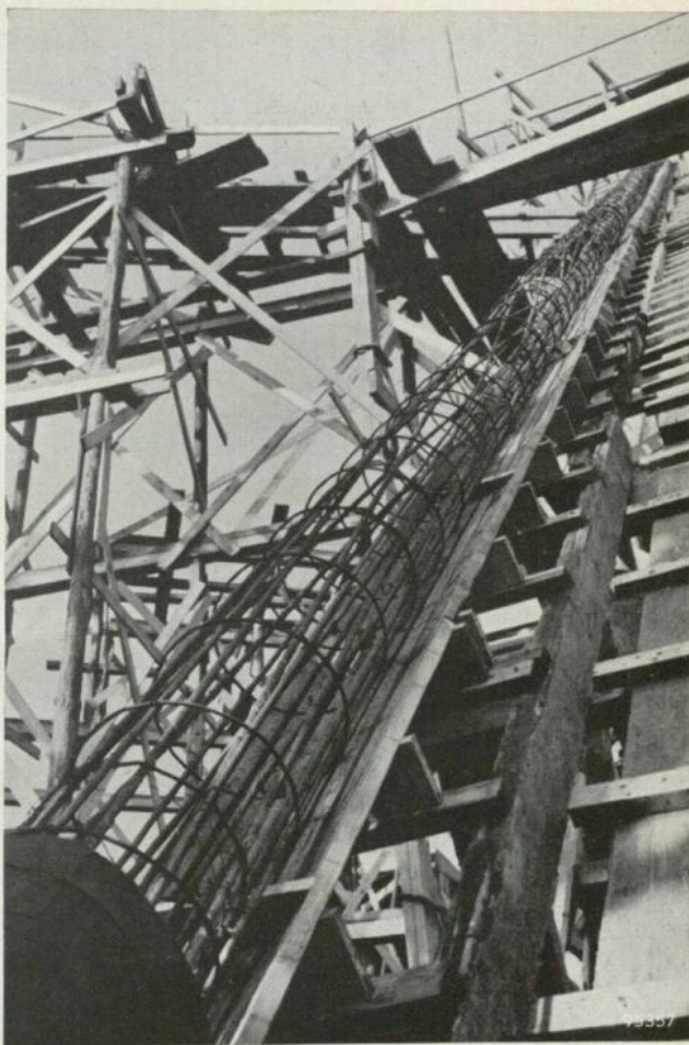
Fig. 9. Prestressing wires for a rib, mounted before making the shuttering and casting the concrete. This particular rib was fitted only with wires for producing torsional prestressing (eight wires running on the circumference of a cylinder, 35 cm in diameter, formed by a series of iron hoops). The 9 mm wires look thicker here since they have been coated with a preparation to prevent bonding with the concrete.
