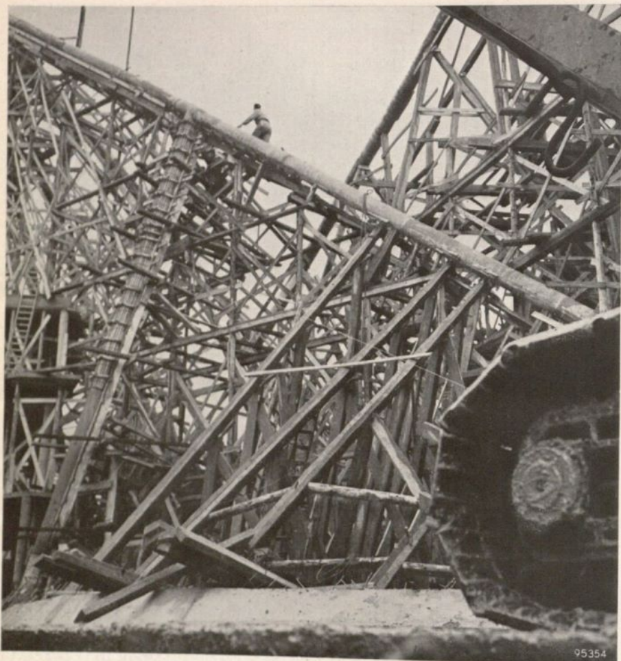
Fig. 4. The 40 cm thick cylindrical ribs were cast in situ in "shuttering" erected on scaffolding.
