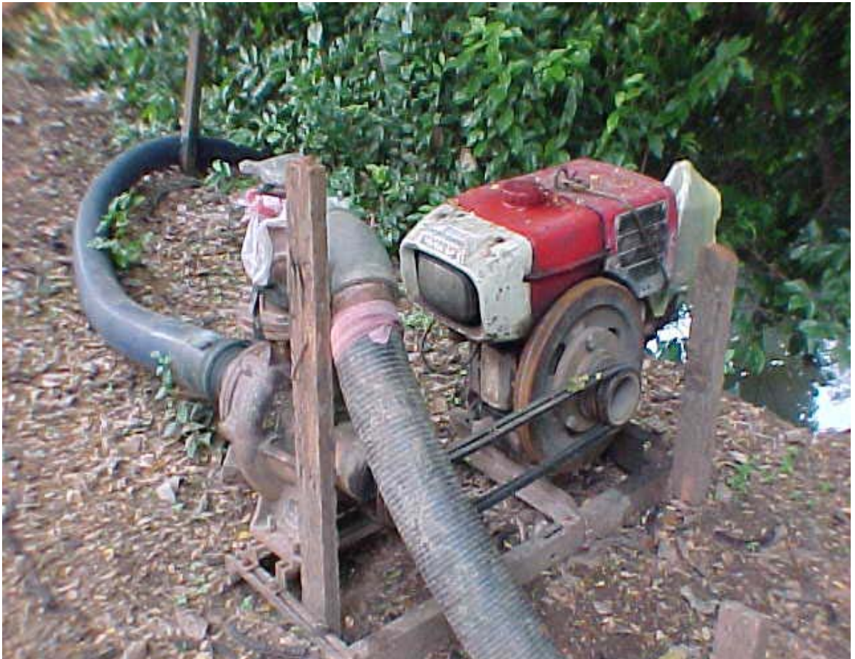
Figure 4--Engine for irrigation pump
